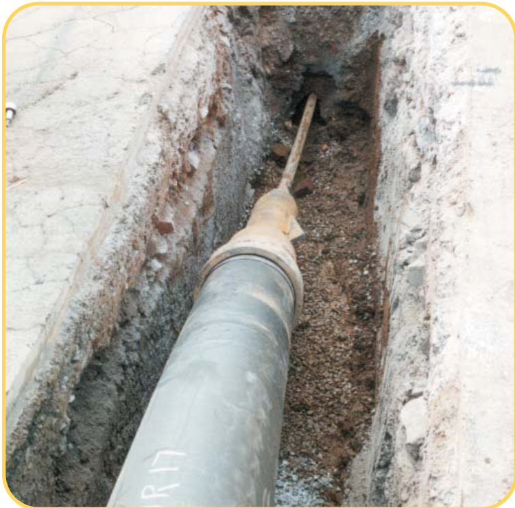
Above: The Impactor with replacement HDPE pipe attached at the start of the burst. Right: The D33x44 Navigator positioned to drill down to the receiving manhole and out through the pipe to be replaced. Inset: The Impactor shown here being extracted from the receiving manhole.
