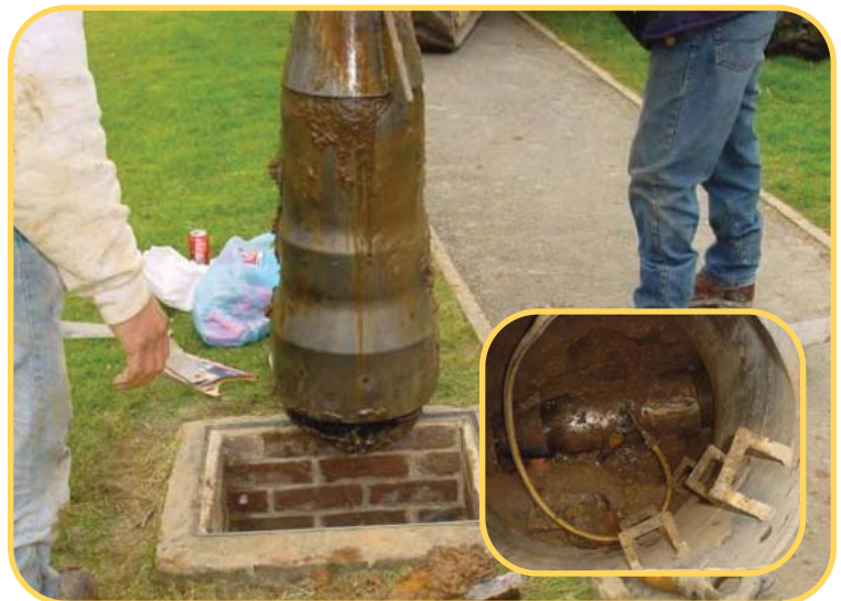
Top: The Navigator D33x44 in place and ready to push rod through the old pipe. Middle: Impactor with new pipe positioned to begin the burst. Bottom: Extracting the Impactor from the end manhole. Inset a view of Impactor entering the manhole.
