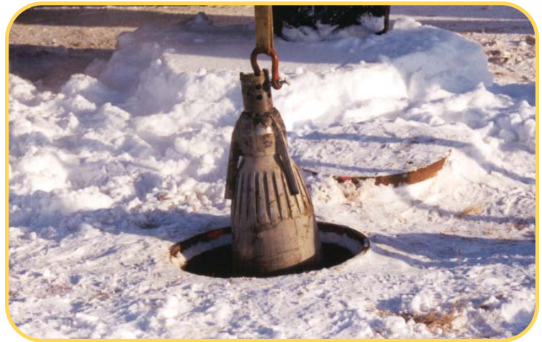
Bottom left: New pipe being pulled in behind the Impactor. Top right: Jon Markel, Vermeer North Dakota, drilling out to the pipe entry point. Bottom right: The Rotary Impactor being extracted from the exit manhole.
