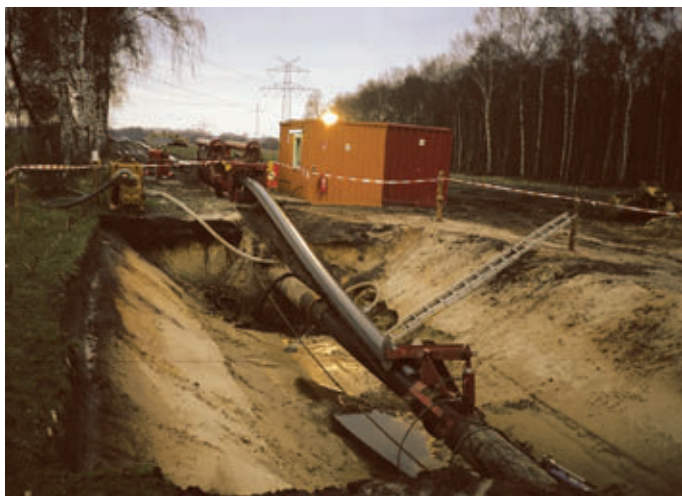
Photo showing PE pipe exiting the heating unit and disappearing into the old pipeline. Special heaters warmed the PE liner before it was reduced and pulled through the old pipeline.
