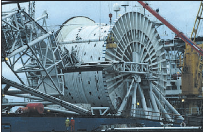
Polyethylene-lined pipe sections are welded and reeled onto a 21-ft diameter reel on the Norlift.
