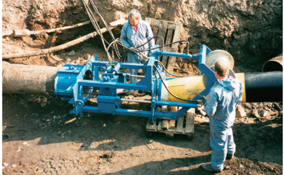
The towing cable and nose cone pass through the Swagelining die as the first installation begins.
