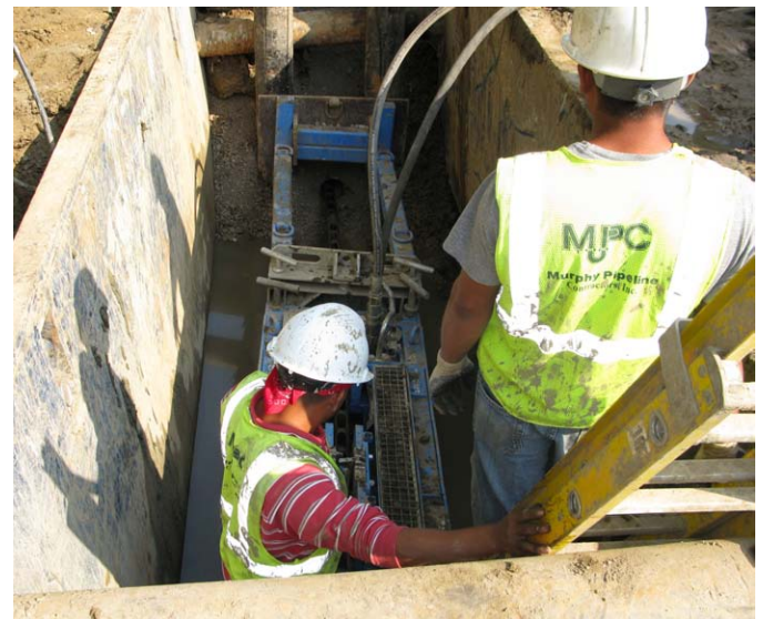
Murphy Pipeline crews employ pipe bursting to install a new 200mm HDPE water main.
