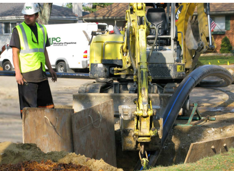
120 meters of new 200mm HDPE enters the launch pit to replace an existing 150mm Cast Iron water main.
