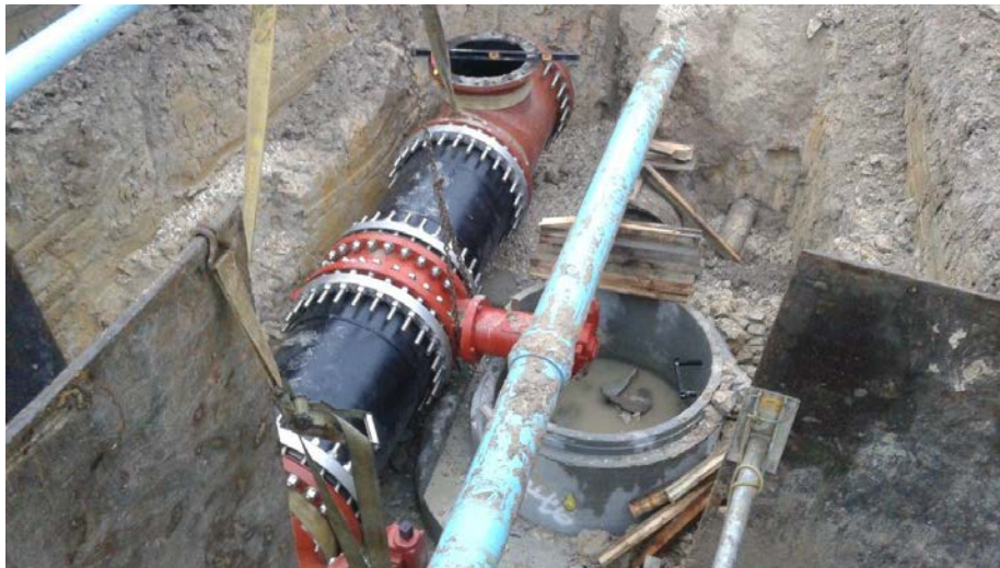
Figure 3: 30-inch diameter butterfly valve with 48-inch operator manhole.
