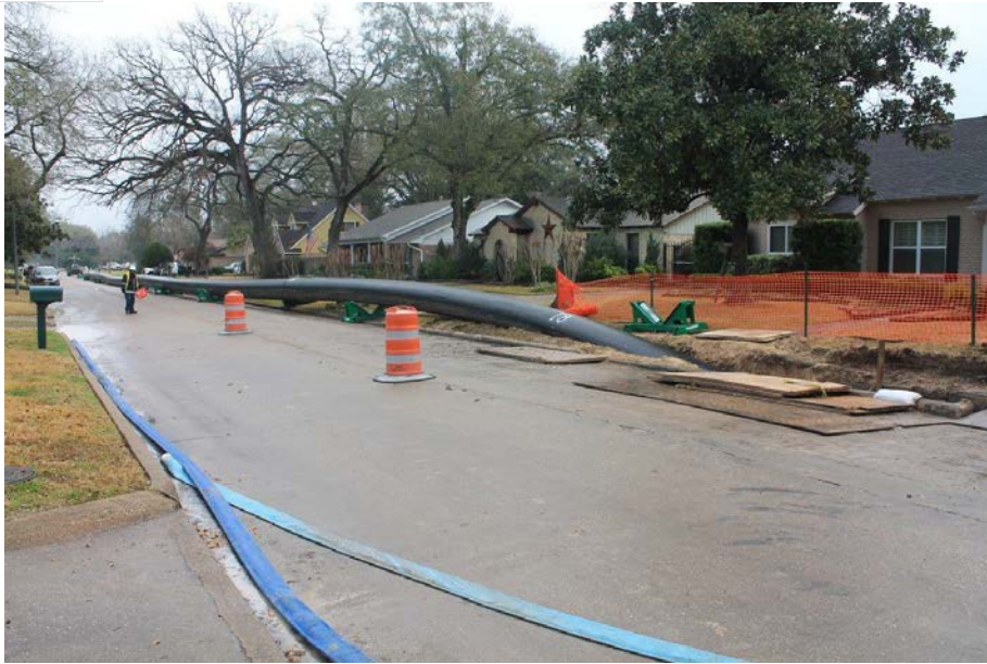
Figure 2: Residential area with limited ROW and mature landscaping. 30-inch HDPE pipe enters insertion pit.
