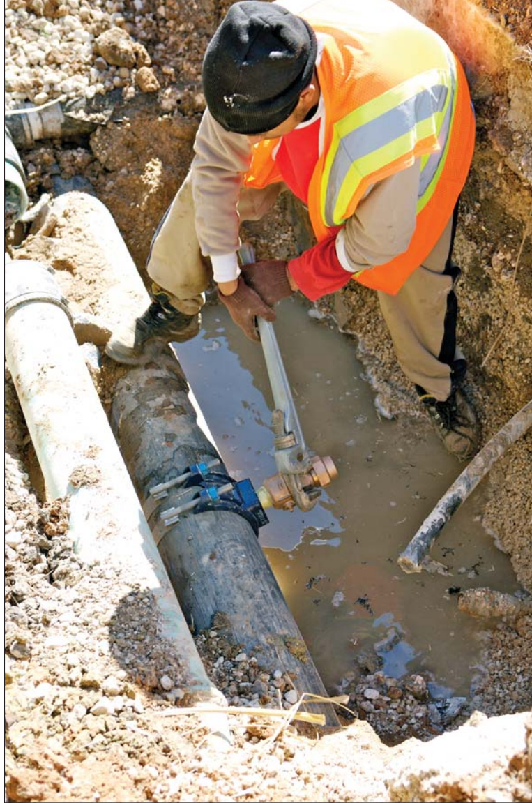
A member of the service crew works to attach a service line to a newly installed main using a mechanical service saddle.
