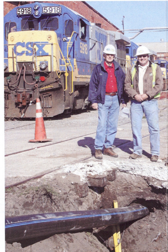
Robert Bates Jr., RBA Inc. Consulting Engineering president and principal engineer, left, and Andy Mayer, Murphy Pipeline Contractors Inc. president.
