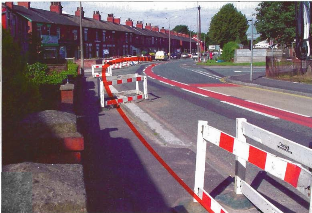
Because the trenchless method was used, disruption was kept to a minimum.
