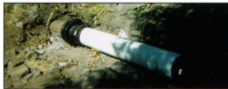
Adjacent sections of lined pipe were bridged by a new steel pipe which was joined to the lined pipe with special couplings.
